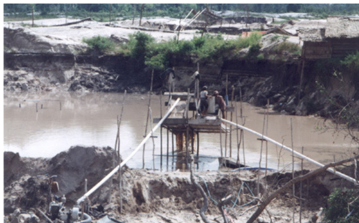
Retaining dam: Water is released from here into the local river system.
